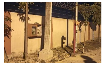
FIRE SAFETY SERVICE
