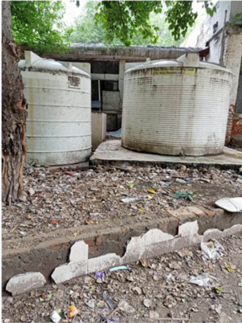
WATER STORAGE TANK
